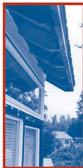
Open eaves, vents not screened (6 pts)
